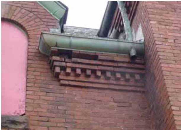
Figure 22. Missing and damaged masonry detailing; copper gutters
