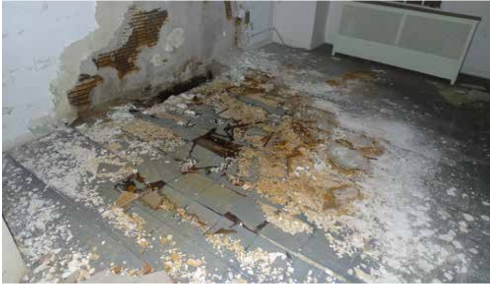
Figure 49. Water damage and deterioration from roof leak
