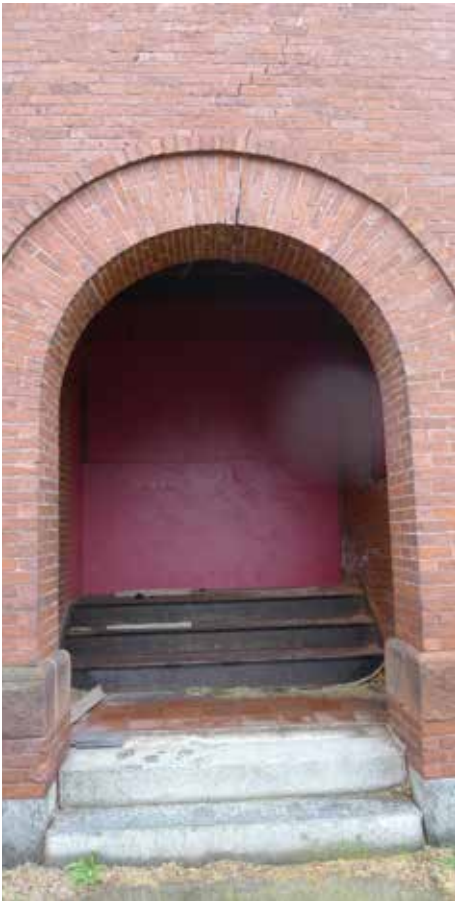
Figure 23. Recessed entry; settlement cracking above brick arch
